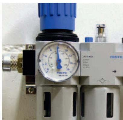
Fig. 2 Deoiler for compressed air
