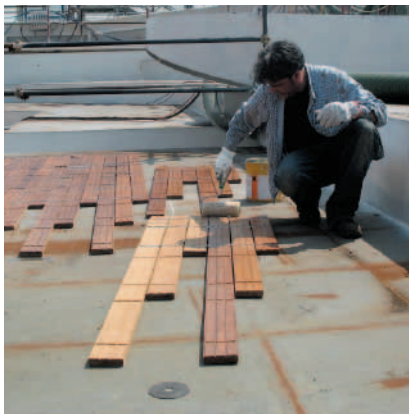
Fig. 9 Applying Sika® MultiPrimer Marine to a teak deck with a roller (hidden side)
