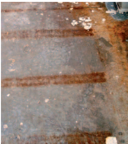
Fig. 2 Typical welds and weld splatter of a steel deck
