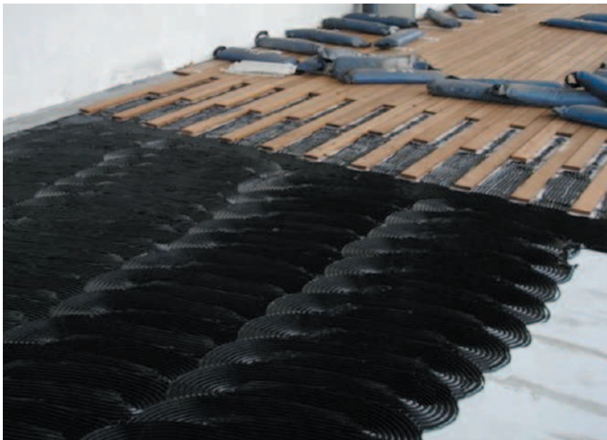
Fig. 14 A teak floor being laid, showing the bedding compound and the weights to hold it in place
